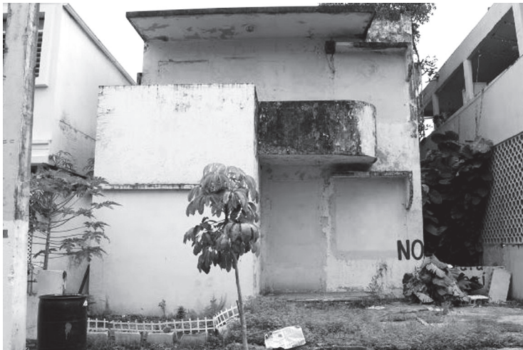
Fig. 4. Casa Taft 169 , San Juan, Puerto Rico, abandoned house, 2013. Photographer: © Marina Moscoso Arabía.
