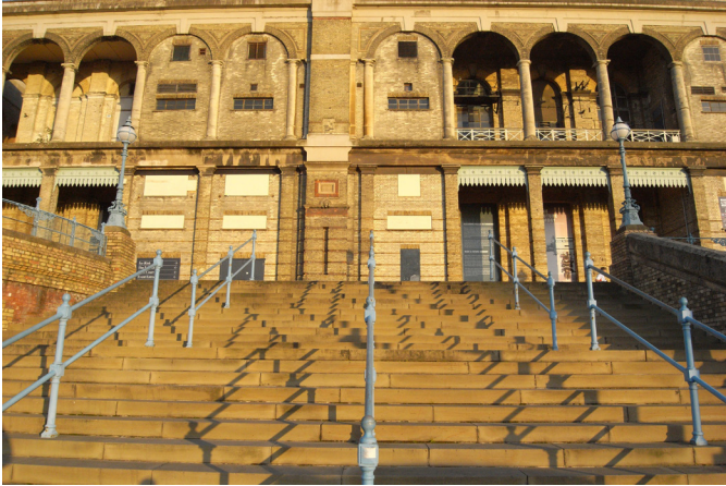
Fig. 4. South façade, main stairs and colonnades, Alexandra Palace, 2014. Image by Rosa Ainley
