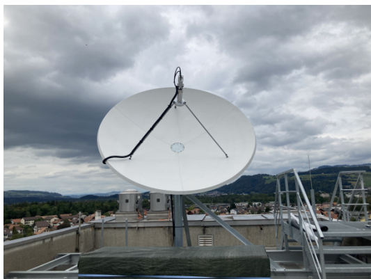
Figure 7. Satellite dish of the downlink ADS-C receiver.
