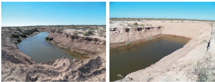
10 La Pasarela project in March 2013 (circled on map). Photo on the left shows the environment upstream of the construction site. Photo on the right shows the construction site
