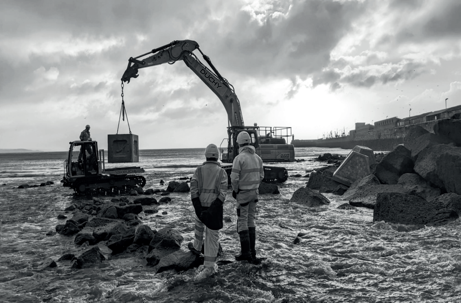
Placement of Eco-blocks along the breakwater at the Newlyn project site. Source: SARCC Project, 2022
