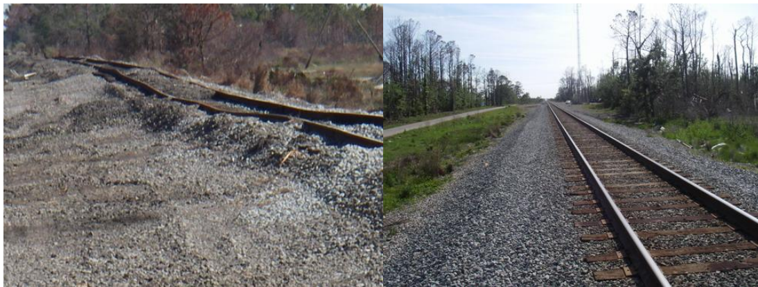
Figure 3. Port Bienville, Mississippi. Left (Oct 2005): CSX railroad, with ballast scoured seaward. Right (May 2006): CSX railroad, repaired.
