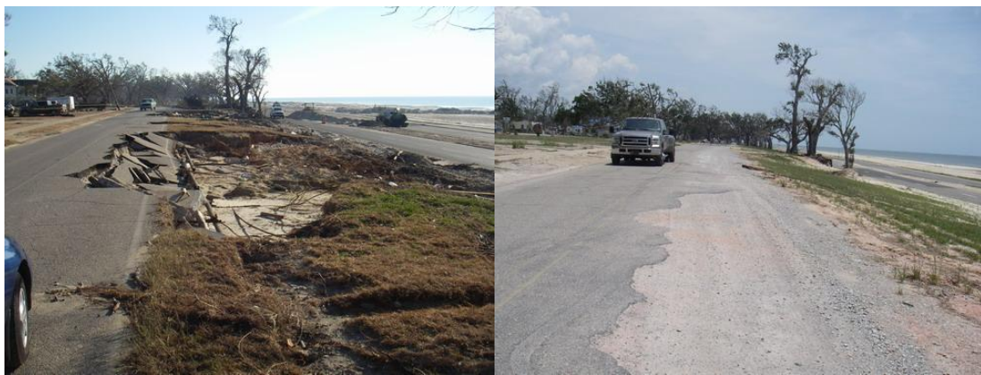
Figure 7. Pass Christian, Mississippi. Left (Oct 2005): Wash-outs along the coastal road. Right (May 2006): Temporary repairs to the coastal road, with gravel.
