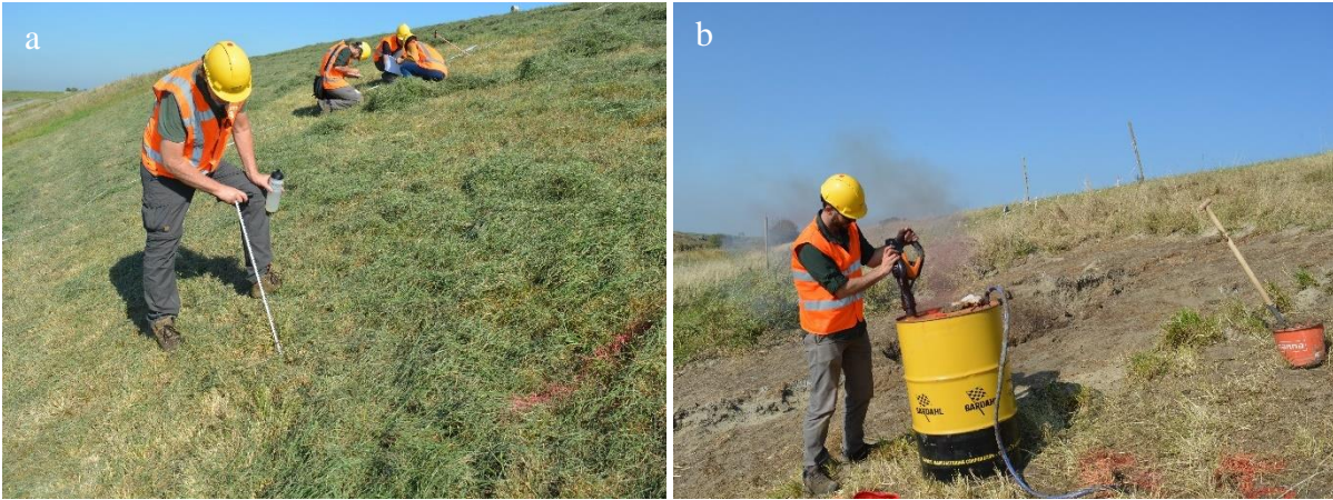
Figure 7: (a) A probe was used to measure the depth of the burrows during the visual inspection of the levee. The burrow openings were not clearly visible because of the vegetation. (b) The smoke test was performed using configuration 1: with a leaf blower the smoke is blown from a container through a hose into the burrow network.
