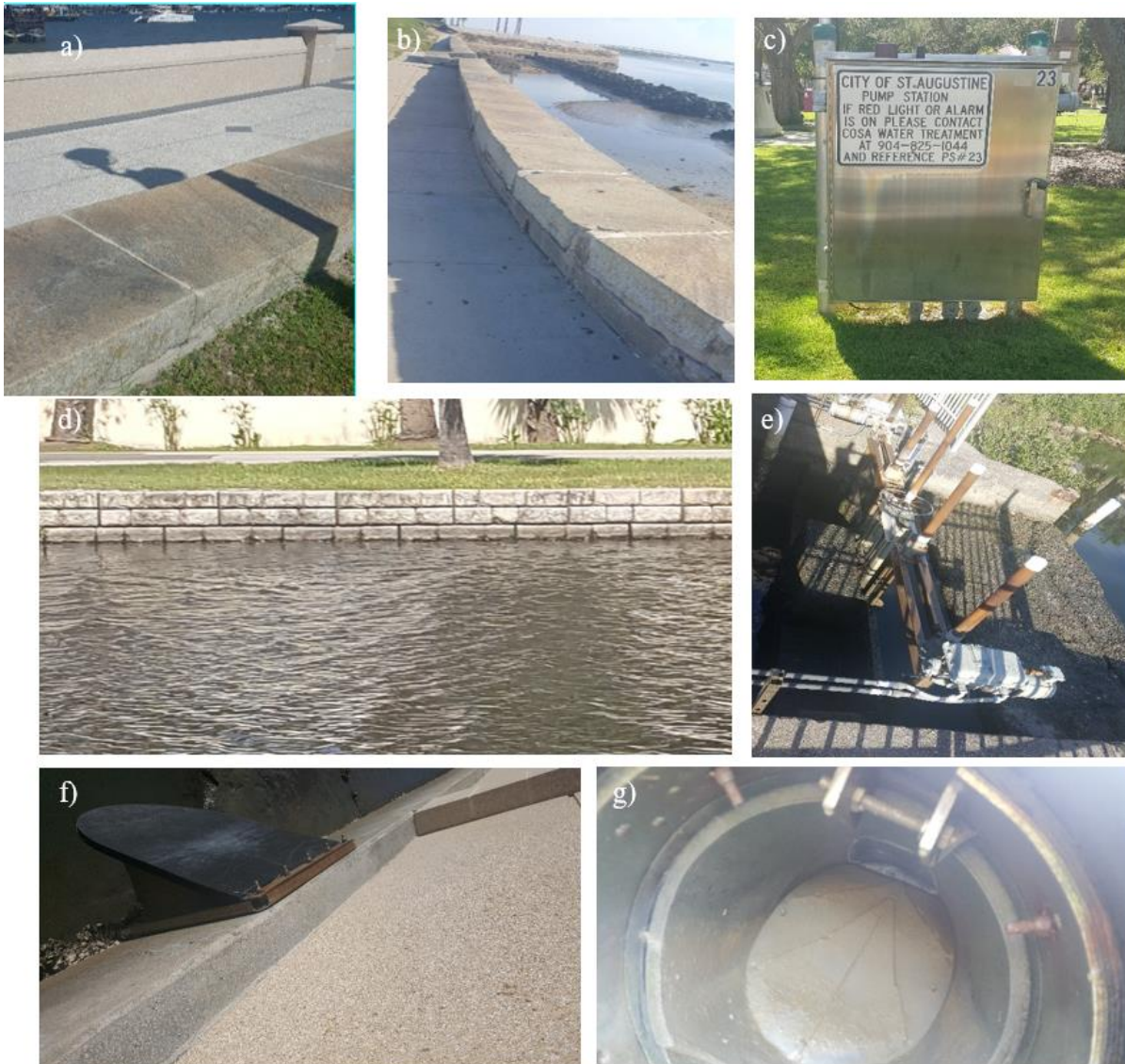
Figure 2. a) New seawall built in 2014 (showing also the old seawall from the 19th century). b) A section of seawall not yet updated. c) A sewage control box which failed when flooded during hurricane Matthew. d) Reinforced walls of drainage lake. e) Site of overflow control for drainage lake, which is slated to be upgraded. f) Previously used flapper outflow. g) Duck bill valve (replacing earlier flapper valves)
