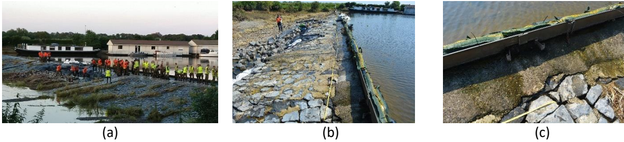
Figure 10: Barrage near Bosscherveld: (a) emergency repairs with the assistance of the army (photograph Wilbur van Beijnen, Directorate-General for Public Works and Water Management), (b) overview of defence after repair (high-water marks still visible from the vegetation in the background), (c) detail of anchoring of steel edge.
