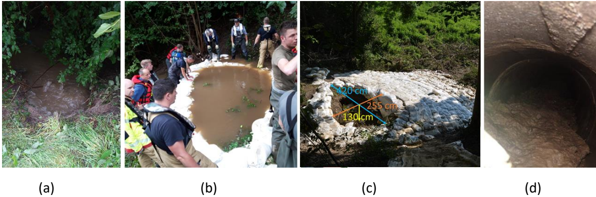
Figure 14: Situation near Bunde: (a) prior to effective measures (photograph Bertram de Rooij, WUR/Fire Service Gelderland Midden), (b) stabilised boiling (photograph Hoite Detmar, the Directorate-General for Public Works and Water Management), (c) boiling area with dimensions after drying out, (d) the concrete culvert where the water came out (photograph Anton van der Meer, Deltares).
