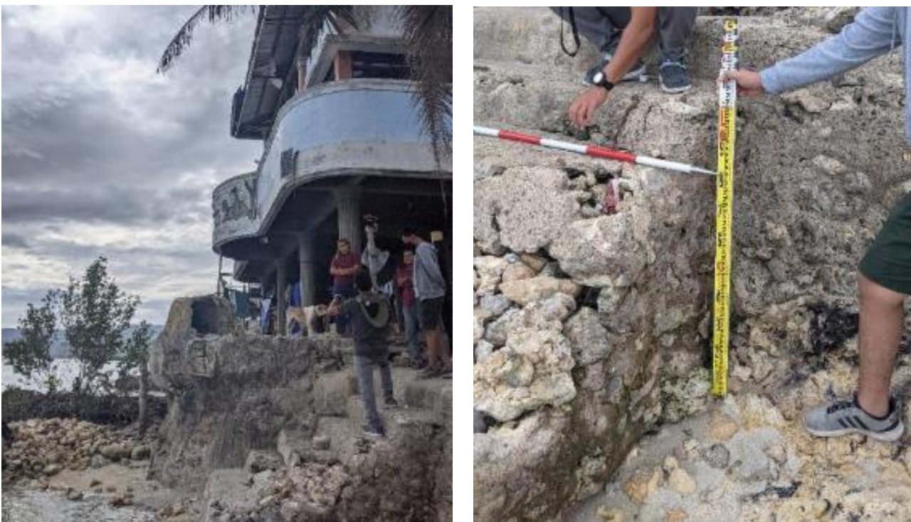
Figure 5. Left. Minor damage to houses located right next to the waterfront. Right. The storm surge only reached the middle of a small staircase used to reach the beach.
