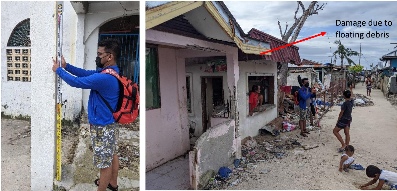
Figure 13. Left. Flooding level in front of the church of Isla Batasan. Right. Damage on edge of a roof due to floating debris.
