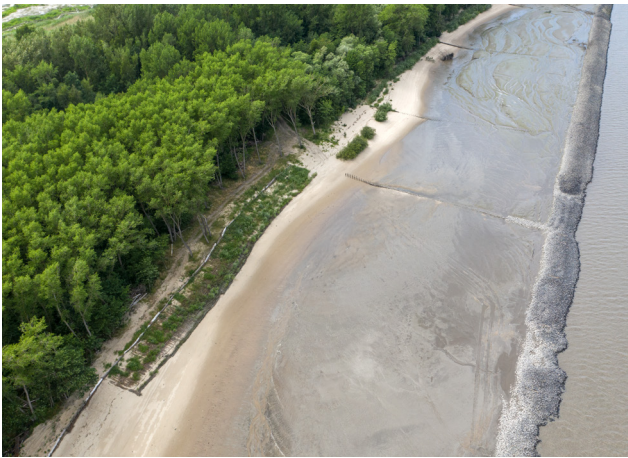
Figure 10: Combination of rubble mound training wall, brushwood fences and live willow staking for embankment erosion control at Hanskalbsand in the Lower Elbe Estuary, Germany. Source: Federal Waterways Engineering and Research Institute (BAW).
