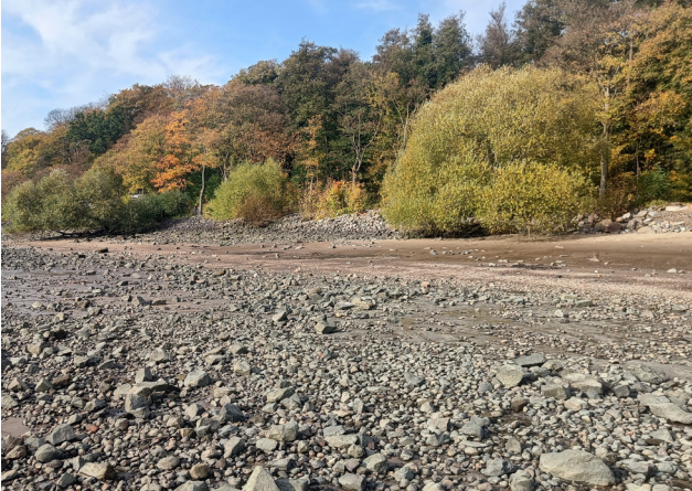
Figure 3: Displacement of rock armour from revetment due to long-period vessel wave action in the Lower Elbe Estuary, Germany. Source: G. Melling.
