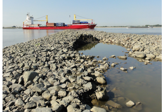
Figure 4: Rock groyne damage due to long-period vessel wave impact in the Lower Elbe Estuary, Germany. Source: Federal Waterways Engineering and Research Institute (BAW).
