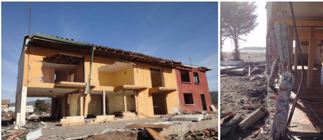
Figure 1: Global (left) and local (right) structural damage (Palermo et al. 2012).
