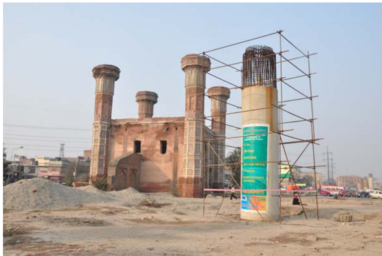
Figure 6 The Orange line construction near the Chaurburji, Lahore (Source: Pakistan Today newspaper)
