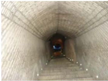
Figure 6 Underground water reservoir (Author)
