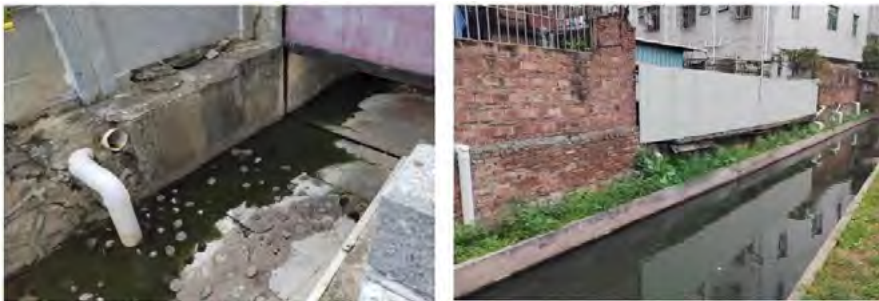
Fig. 13 & 14. Comparison between the renovated and unrenovated runoff
