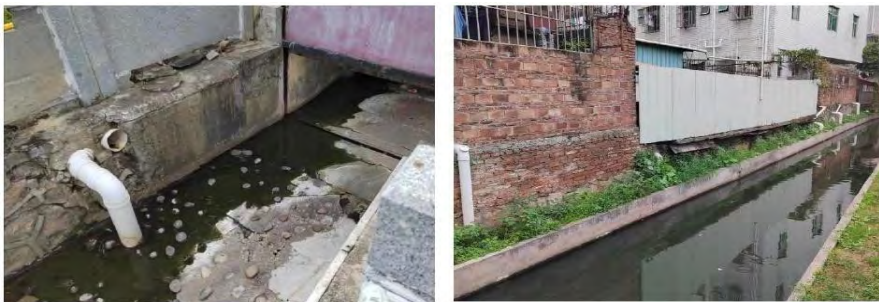
Fig. 13 & 14. Comparison between the renovated and unrenovated runoff
