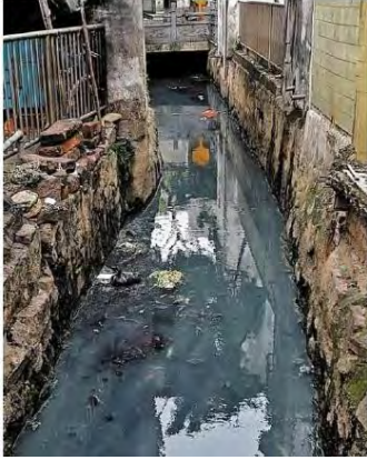
Fig. 5. Longjin River before the renovation. The Longjin River prior to the renovation exhibited black and malodorous water.
