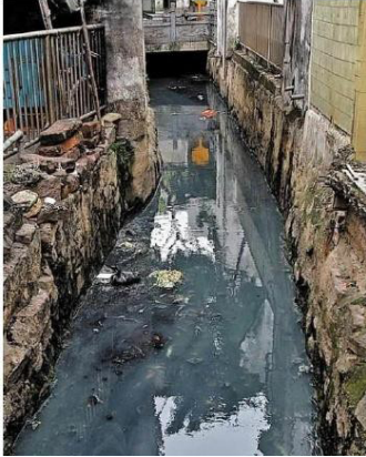
Fig. 5. Longjin River before the renovation. The Longjin River prior to the renovation exhibited black and malodorous water.
