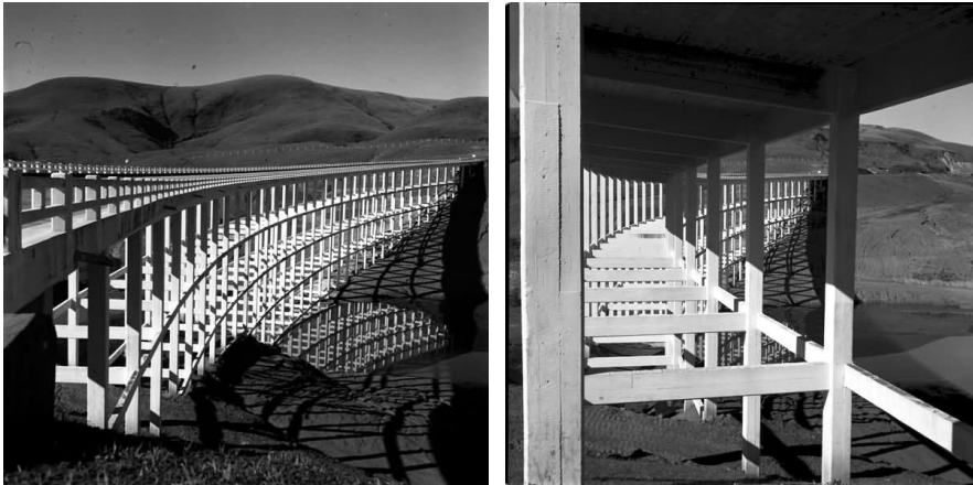
Fig. 5. Viaduto Vila Rica, 1957. Originally named the Viaduto das Almas, this viaduct spans the Córrego das Almas, a tributary of the Velhas River. Located on the BR-040 highway, connecting Rio de Janeiro to Brasília, it is 50 km from Belo Horizonte and has a length of 262 meters..
