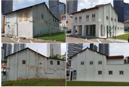
Shophouses at 45 Sultan Gate before and after restoration, the first state properties to be launched for tender. PHOTOS: SLA
