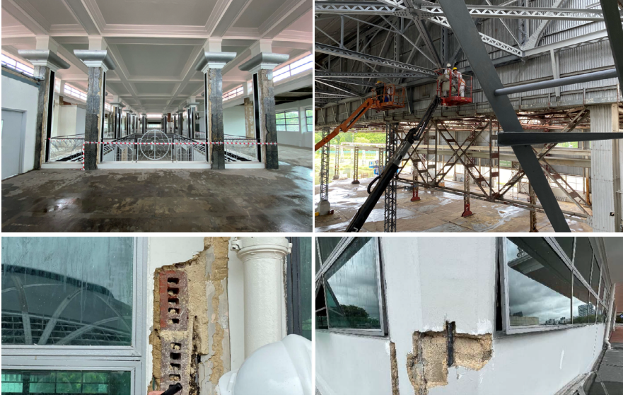
Fig. 13. Clockwise (L to R) - Level 2 of Terminal Building with exposed columns, Workers in the midst of repainting steel trusses of Hangar A, External wall of Terminal Building stripped of plaster exposing brickwork, External wall of Terminal Building stripped of plaster exposing block masonry, reinforced concrete structure and embedded piping. (Source: DPA)
