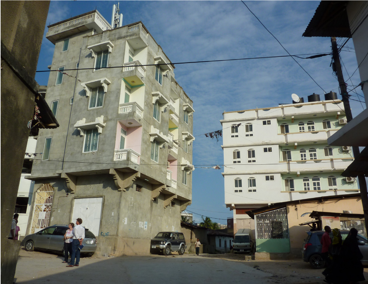
FIGURE 6 A typical example of recent postmodern multi-storied Swahili houses in Kisimamajongoo, Ng'ambo.
