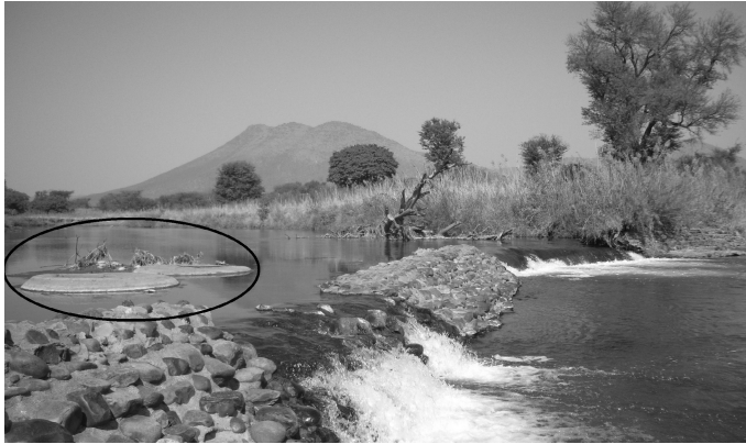
Figure 5. The pumps in the Steelpoort River supplying water to GaManoke ©Richard Meissner
