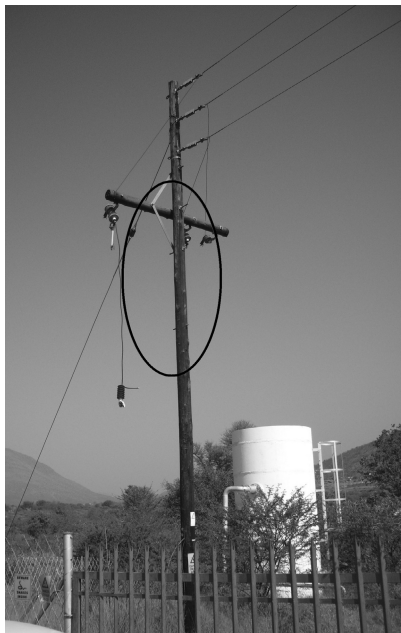
Figure 6. The missing transformer at the GaManoke water purification plant ©Richard Meissner
