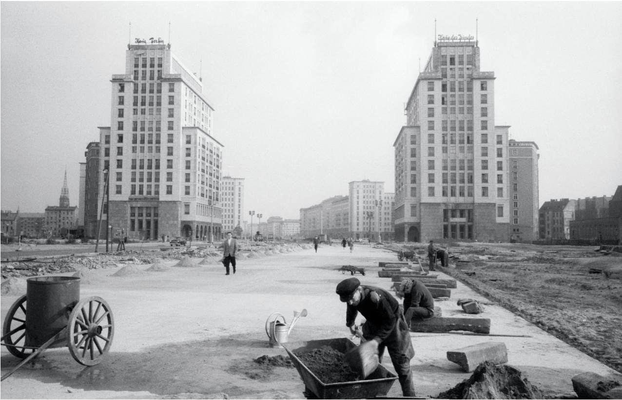
Bouw van de Stalin-Allee (nu: Karl-Marx-Allee) in voormalig Oost-Berlijn Construction of the Stalin-Allee (now called Karl-Marx-Allee) in the former East Berlin
