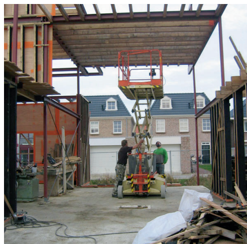
De bouwlift die later een plek kreeg in de villa The builder's hoist which later was incorporated in the villa
