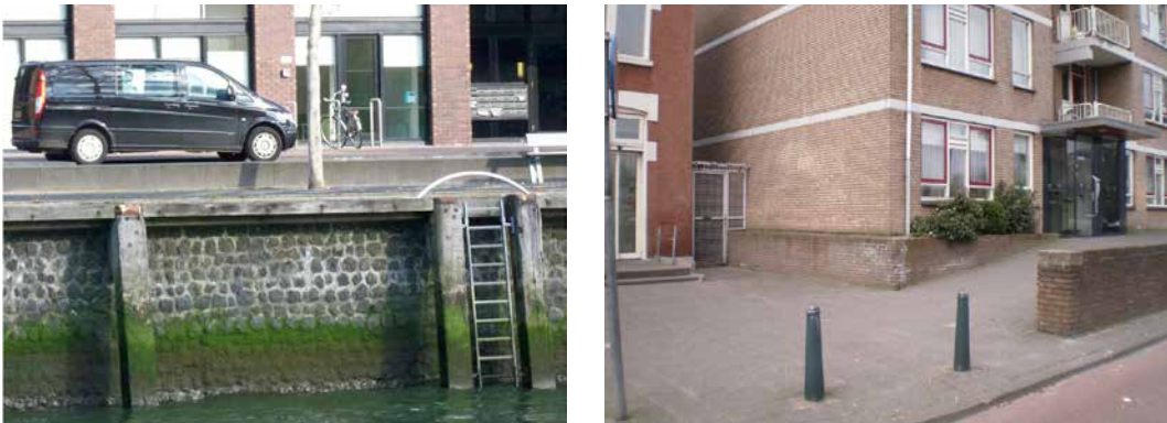
FIGURE 4.9 Left picture: land elevation at an urban development of the former port area in Rotterdam (Müllerpier). Note that the land elevation keeps a distance from the bulkhead to avoid structural integrity problems of the historical quay construction. Middle picture: elevation of an infill building (Feijenoord, Rotterdam). Photos by author.
