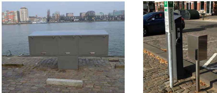
FIGURE 4.15 Elevated shore power supply facility in Dordrecht, The Netherlands (left) and flood protected power distribution station at the Noordereiland, The Netherlands. Photos by author.
