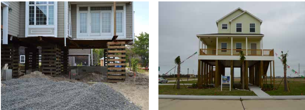
FIGURE 4.13 Left: elevating of an existing wood frame building above flood elevation level, Jersey Coast, New Jersey, US. Picture right: new constructed waterfront property on Galveston Island, Texas, US. Photos by author.
