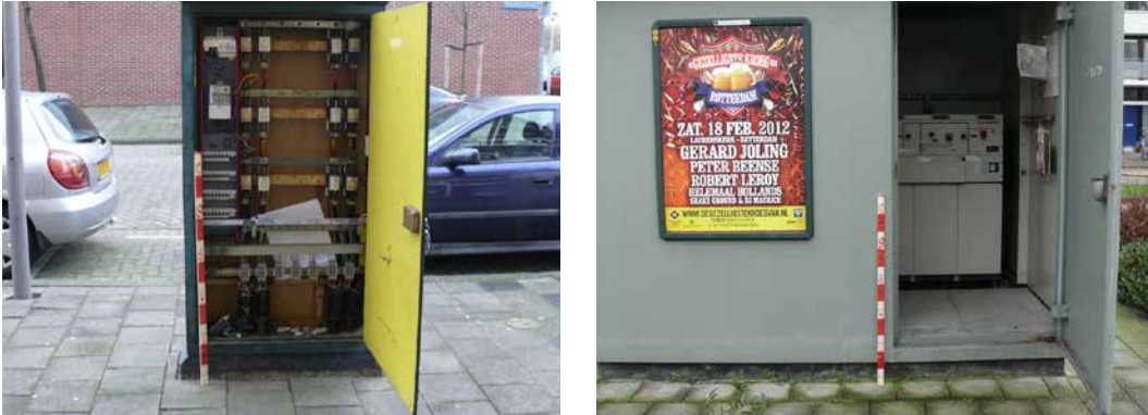
FIGURE 5.3 Typical low voltage (left pictures) and medium voltage distribution stations (right picture) at Rotterdam. Critical threshold of these cabinets is an inundation that reaches depths of 30 and 50 cm respectively. Photos: Robert de Kort (2012).
