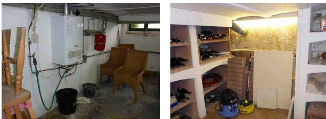
FIGURE 6.4 A substantial part of the costs of flooding of residential buildings is due to the vulnerability of building systems, interior and storage of sensitive goods in basements. Photos: Kuijk & Boer (2015).
