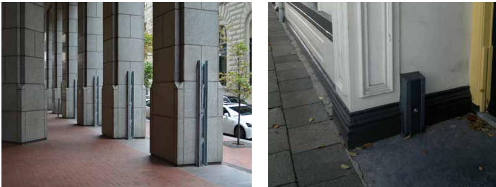
FIGURE 4.10 Example of retrofitting dry proofing to an existing office building in Manhattan, New York (left) and an historical building in Kampen, The Netherlands (right). Both dry proofing solutions are based on installing panelised flood protection during high water conditions. Photos by author.
