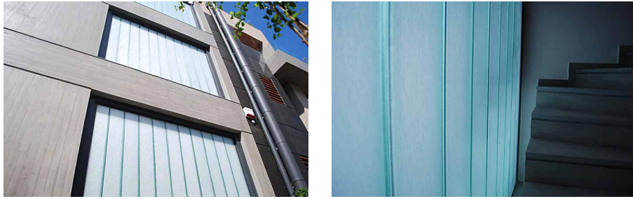
FIGURE 6.4 Translucent insulation used in the façade of the staircase of a private dwelling in Filothei, Athens, Greece by GEM architects. Reprinted from Helmania website.
