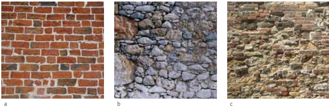
Figure 2.6 (a) Clay brick wall in Germany, (b) masonry natural stone wall in Greece, (c) wall with stone and brick mixed construction in Czech Republic.
