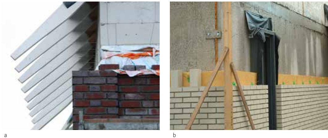
Figure 2.9 Current construction of an external wall with facing bricks, lime stone (a) or concrete (b) backing wall and insulation in the cavity
