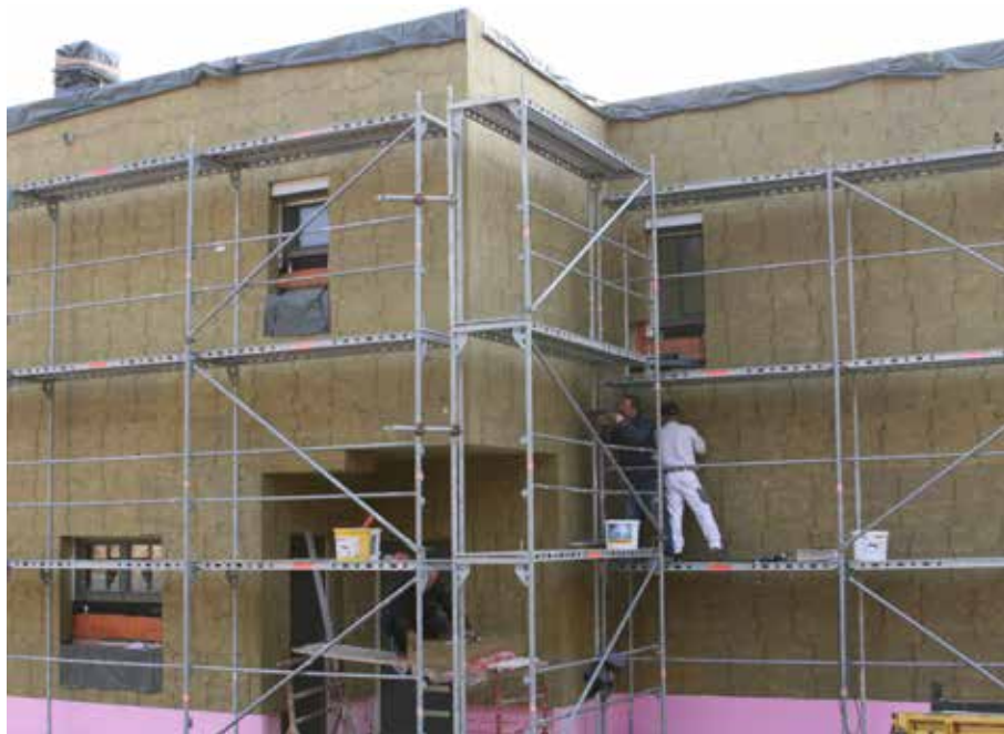
Figure 4.11 Application of insulation externally on the wall (Image source: courtesy of ROCKWOOL International A/S).
