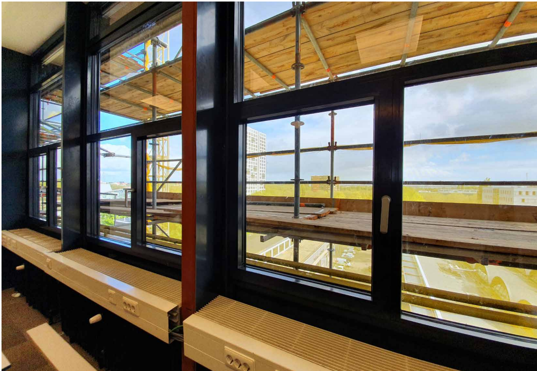
FIG. 5.1 Interior photograph of the FaaS façade renovation at the CITG faculty building large-scale demonstrator prototype, at TU Delft, in the Netherlands. (Photo: Azcárate-Aguerre, 2019)
