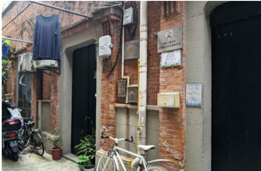
FIG. 8.14 The newly added elements on the façades, such as equipment for fire safety and the white sewage outlets. Source: author, 2018.
