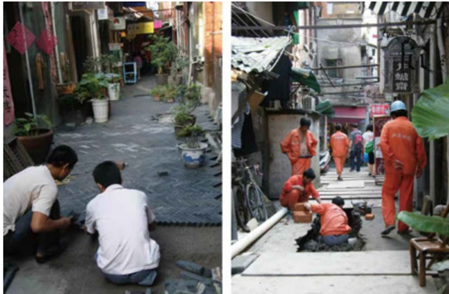
FIG. 7.26 Tianzifang under construction of re-paving (left) and undergrounding pipes (right) in 2009 before the EXPO. Source: Shanghai Shikumen Cultural Research Centre, 2009.
