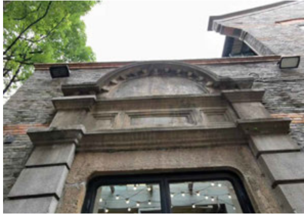
FIG. 6.14 Conserved pediment of the gate frame with obvious patina. Source: author, 2021.
