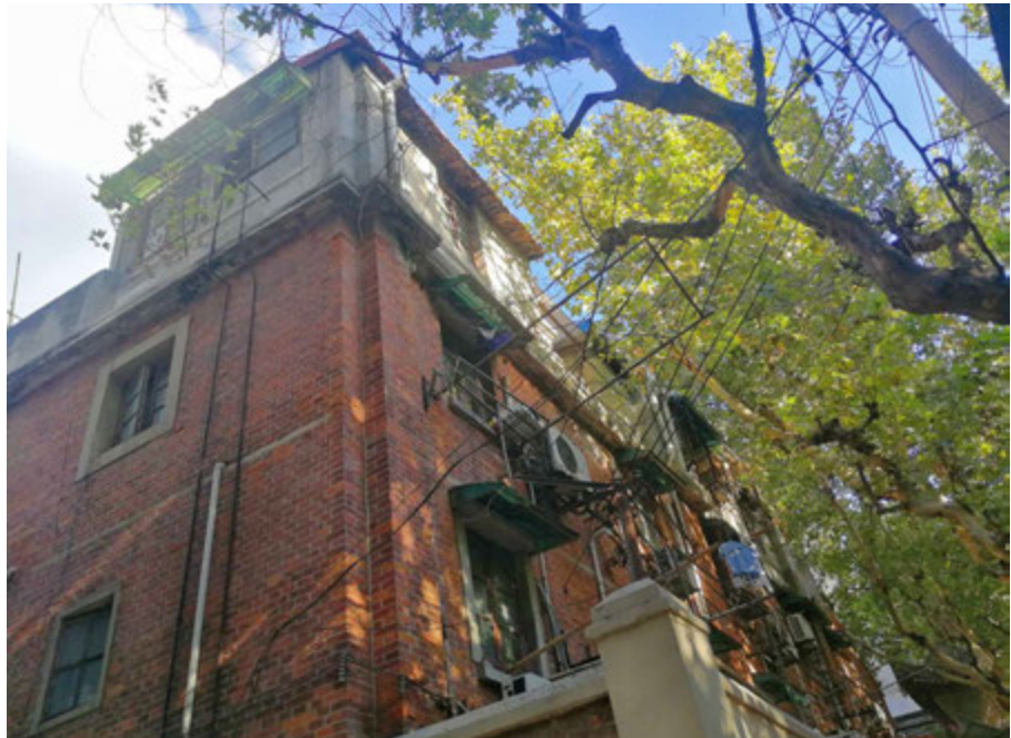
FIG. 8.26 The additional one floor on the top of the original building with grey in colour and plaster in material, replacing the red bricks. Source: author, 2018.
