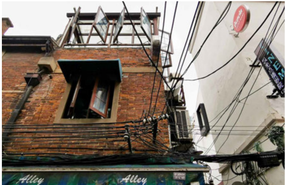
FIG. 7.25 Additional layer of a glass room on the top of the original brick house. Source: author, 2019.
