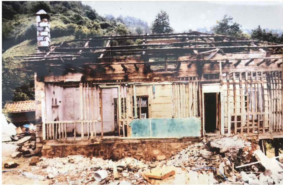
FIG. 4.10 The stones are removed one by one and each of them is given numbers to remember where the pieces belong in the frame. Source: Family archives of Babalik mansion household.
