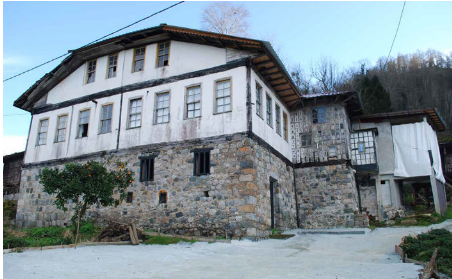
FIG. 6.13 Akyasalar mansion in Çağlayan village grew with the concrete addition. The front façade is plastered, and the addition of stone-infilled timber and the painted addition at the very end with concrete addition reveals the later incompatible constructions. Source: author.
