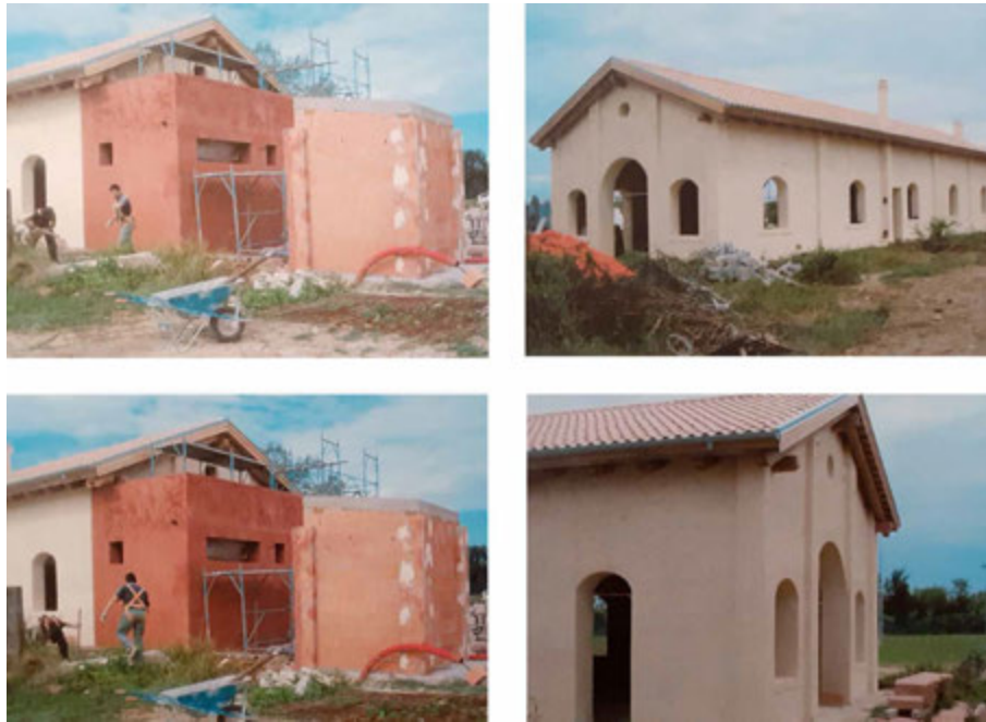
FIG. 5.91 Venice (IT), Forte Cosenz, tool shed: works in progress for the refurbishment of the building (2008) (ASABAPV, Box Mestre: Forti: Forte Cosenz )
