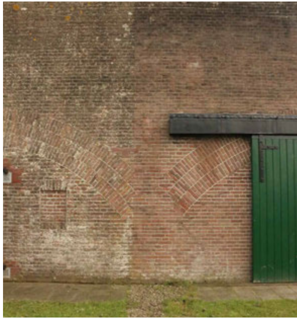
FIG. 4.50 Bunnik (NL), Fort bij Vechten. Bombproof barracks: partial cleaning of the façade in the portion falling within the strook (strip) (F. Marulo 2020)
