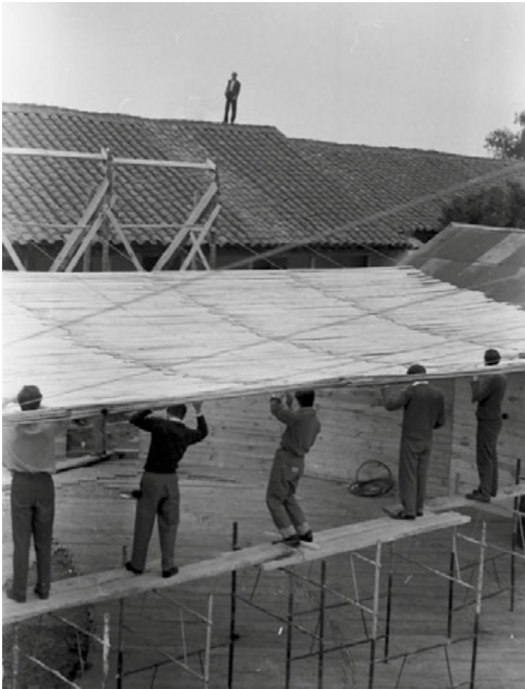
FIG. 4.3 Construction of the pavilion that accommodated the exhibition of the PUCV School of Architecture and Design during the Primera Conferencia Latinoamericana de Escuelas y Facultades de Arquitectura. Santiago, 1959. Archivo Histórico José Vial Armstrong e[ad] PUCV.
