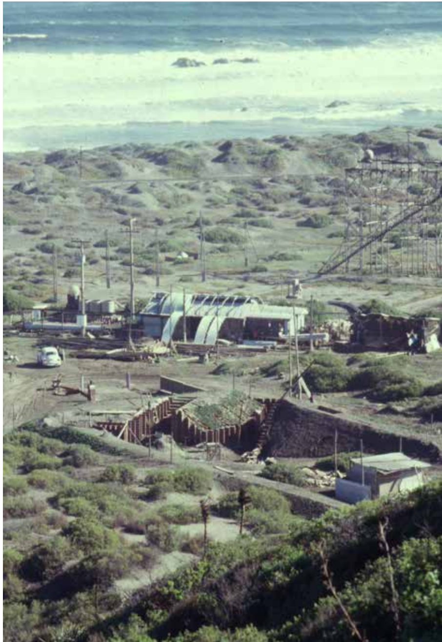
FIG. 1.13 In the foreground, the construction site of the Hospedería de la Entrada , followed by the infrastructure of the construction workshops with its curved roofs, and in the background, the water towers. Ciudad Abierta , ca. 1973. Source: Archivo Histórico José Vial Armstrong e[ad] PUCV.
