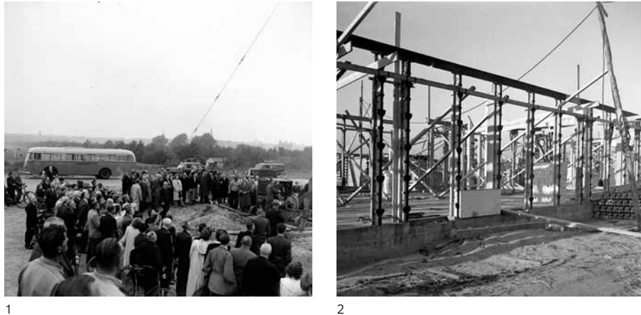
FIG. 7.18 [1] The Social-Democrat alderman for both Housing and Public Works, Jonas van de Velde, drives the first of 6 000 piles for Tuindorp Frankendaal public housing on 22 September 1949 (N Swaager; SAA: 5293FO000815); [2] The construction of the ground floor of the Frankendaal public housing complex. The first prefabricated concrete Skalja panel has been placed in the middle of the façade. (N Swaager, January 1950; SAA: 5293FO000825).
