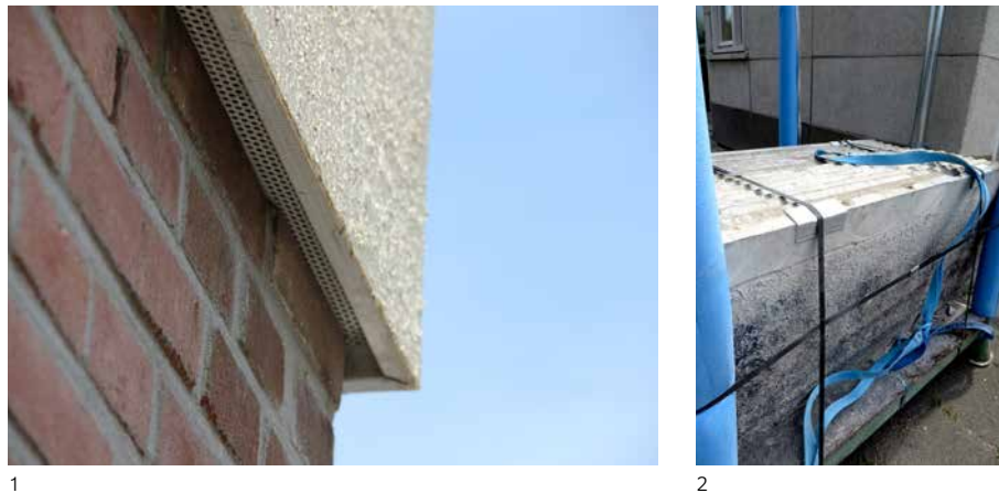
FIG. 7.33 [1] Corner detail of the plasterwork finish on insulation on not-national monuments blocks. The imitation panel finish now stands proud of the brick skin which was already an addition to the end-walls (2018); [2] Repurposed (cleaned and cut-back) prefabricated rain shields, on-site, ready for reinstallation. The circular grinder cut marks on the top left .of the first panel indicate where the upstands have been cut back (2017).
