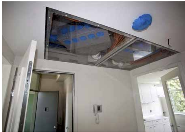
FIG. 6.28 The air handling unit of the demonstration apartment, visible through a transparent ceiling section (Van de Bree & Horst, 2013, p. 17).
