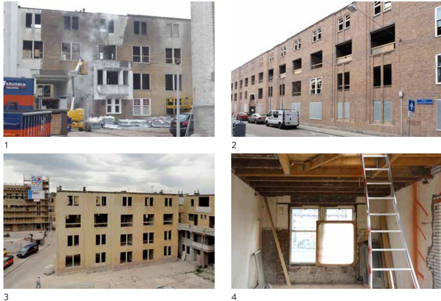
FIG. 5.26 The Justus Quarter renovation project: [1] Steam cleaning the facade (J Molenaar); [2] The Pieter Langendijk Street façade; [3] Inside the block; [4] Interior of a ground floor apartment (all 2011).
