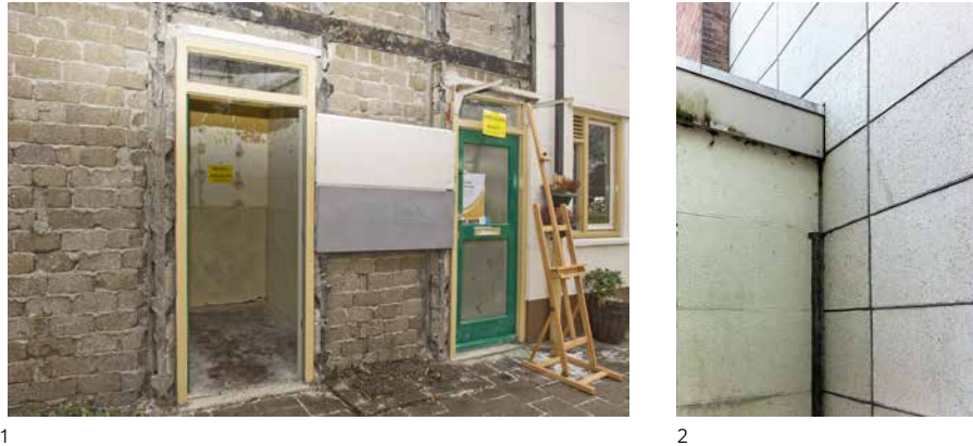
FIG. 7.31 The trial block at 127 Hugo de Vries Avenue with the façade panels removed (Hooysschuur Architects 2010); [2] Connection of the new façade of the trial unit with the unrenovated façade of the adjacent shop (2019).
