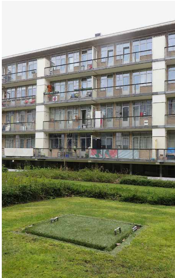
FIG. 6.35 The Koningsvrouwen van Landlust housing complex in 2016 with the cover over aquifer thermal energy storage well in the foreground (2016).
