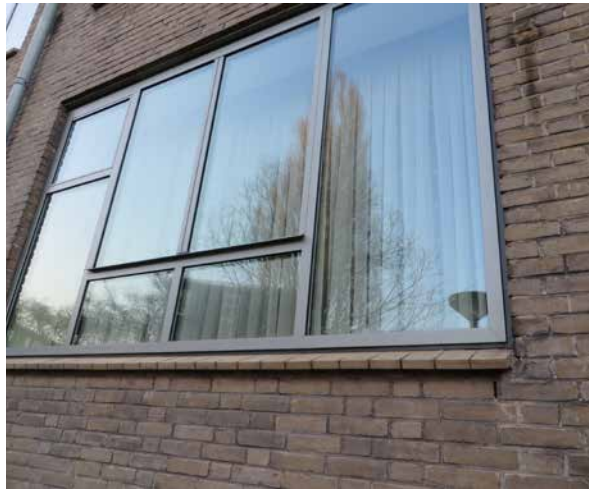
FIG. 6.31 The bespoke "Landlust" window, specially developed to mimick as closely as possible the original steel framed windows, but manufactured from aluminium and with double-glazing (2016).
