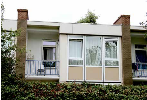
FIG. 7.35 'To do, or not to do'—fuzzy façades of the De Key housing component of the Jeruzalem monument: new timber windows to the balcony, old PVC to the lounge (2018).
