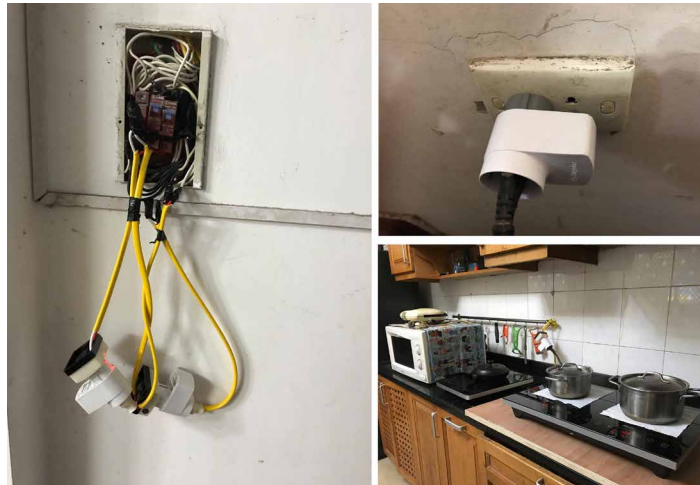
FIG. 7.2 Plug-wise unit installed for energy measurement
