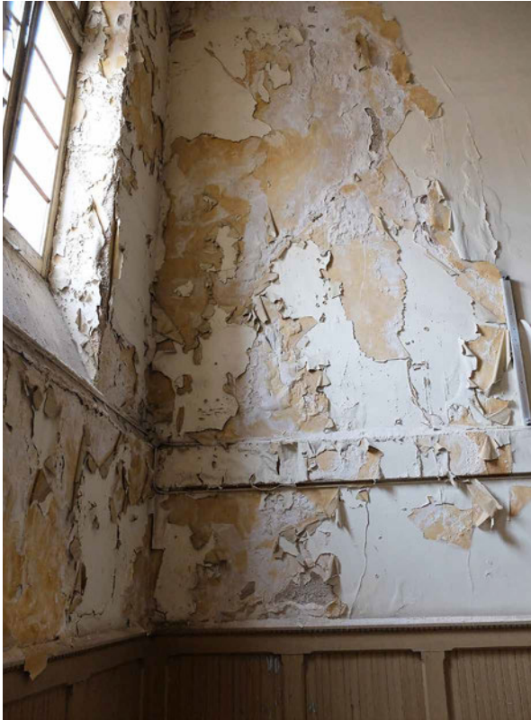
FIG. 14.5 Moisture damage in the central staircase of the Tabacalera, 2017.
