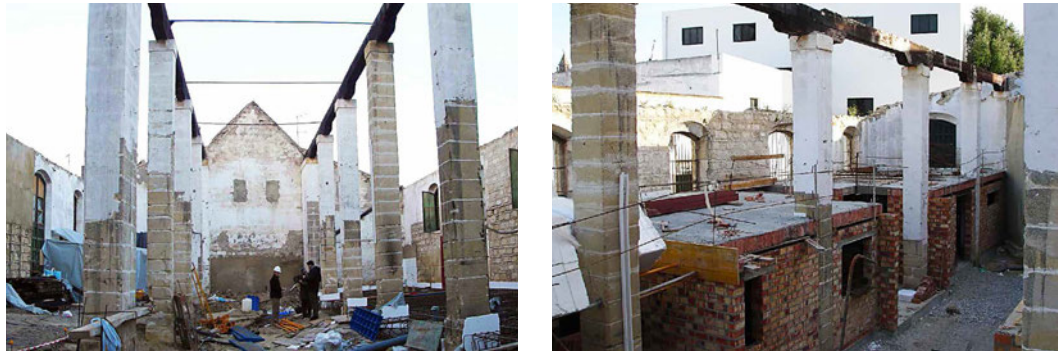
FIG. 12.7 Views of the central patio of the bodega on 11, Liebre st, during its conversion into social housing (Sánchez, 2014, 31-32).
