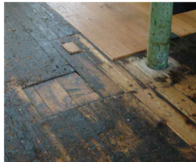
FIG. 3.13 Detail of the floor of the Bell Mill. The original wooden floor boards have been retained where possible, 2015.
