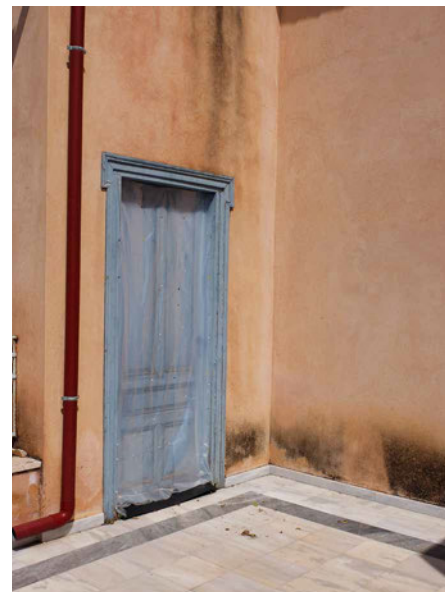
FIG. 18.9 Rising damp and temporary measures for avoiding leakages in the administration building of the LTCP, 2017.
