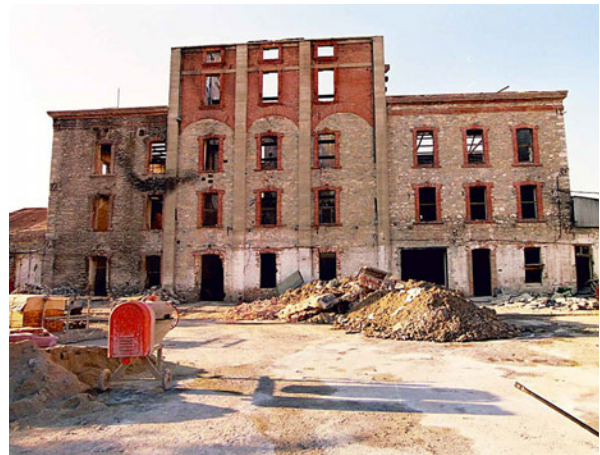
FIG. 20.3 The mill after the fire (Municipality of Larissa - Directorate of Technical Services - Section of New Projects, 2011, 10).
