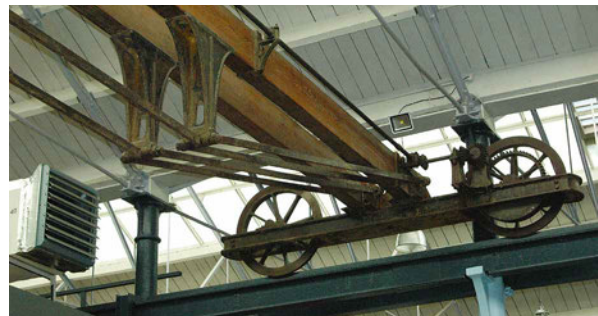
FIG. 2.10 Overhead crane preserved in situ in the halls of the McArthurGlen Designer Outlet Great Western, 2015.
