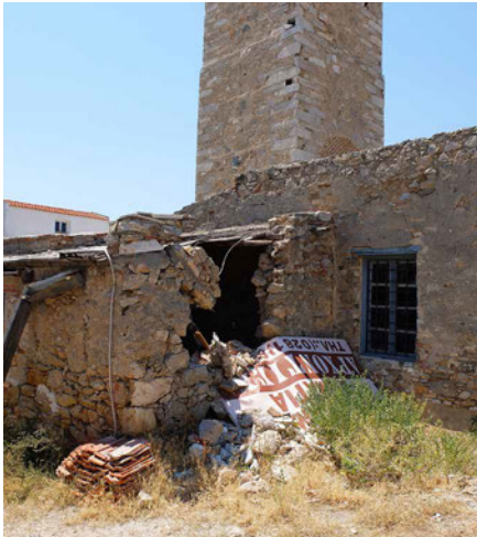
FIG. 16.13 The converted Aneroussis Lead Shot factory in the Summer 2017. The building remains closed to the public due to a partial collapse of a structure attached to it.
