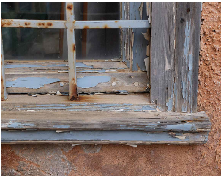
FIG. 18.8 Water damage and signs of corrosion to the windows of a restored building in the LTCP, 2017.
