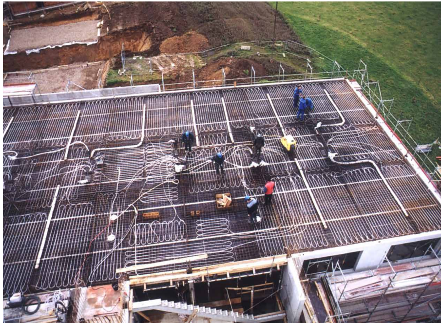
FIG. 1.3 Installation of the Thermo Active Building System in the form of a radiant slab in the Balanced Office Building (BOB) engineered by VIKA Ingenieur GmbH in Aachen. (VIKA Ingenieur, 2005)
