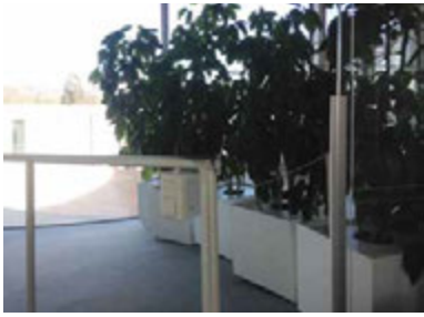
FIG. 5.8.1 Worn railing at barrier to books ...
