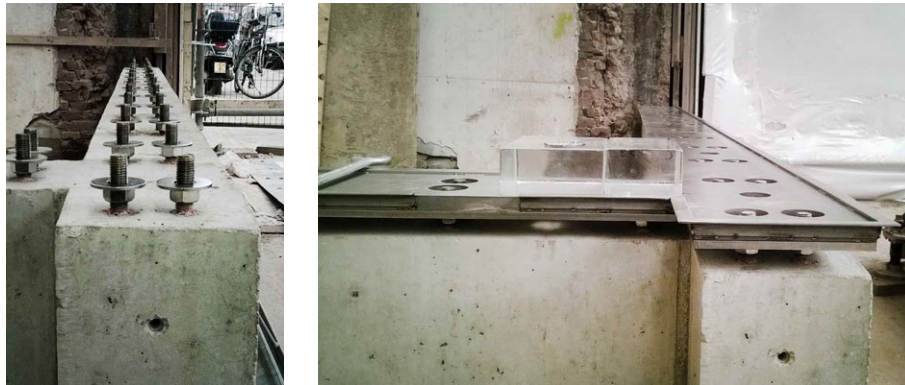
FIG. 6.10 On the left the bolts used for levelling the stainless steel plate, seen on the right.
