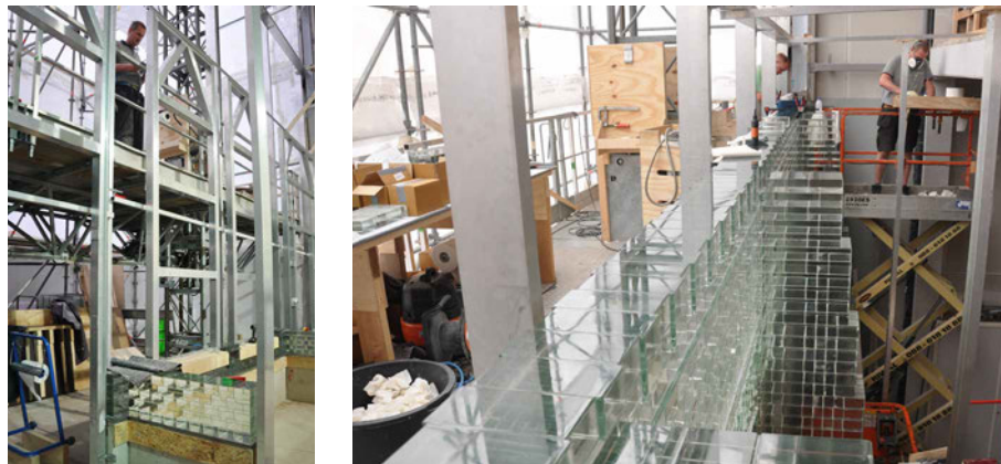
FIG. 6.9 Left: the installed aluminium place holders of the opening. Right: The mast climbing working platform and one of the three mobile elevated platforms.
