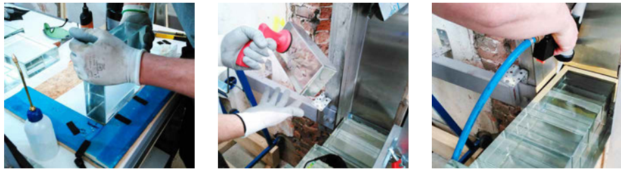
FIG. 6.21 From left to right: Bonding of the steel plate to the corner brick. Positioning of the brick by a suction cup holder. Application of the semi-elastic polymer.
