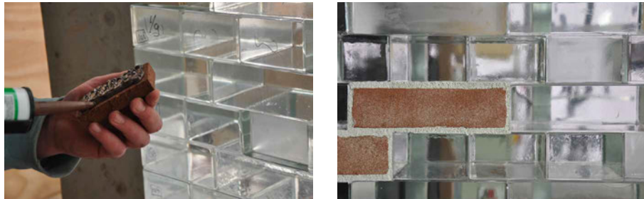
FIG. 6.19 Left: Bonding of the ceramic strips to the shorter bricks. Right: The final visual result.
