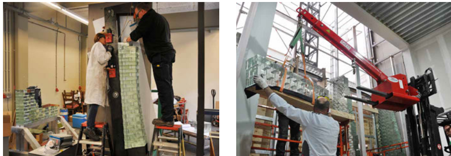
FIG. 6.17 Left: The special rotating fixture for the preassembly of the architraves. Right: The installation of the bonded architraves on site.
