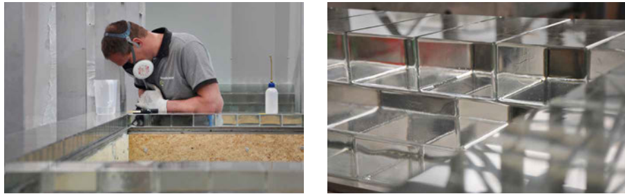
FIG. 6.15 Left: Sealing of the already bonded bricks. Right: the final, visual result achieved by the novel bonding method.
