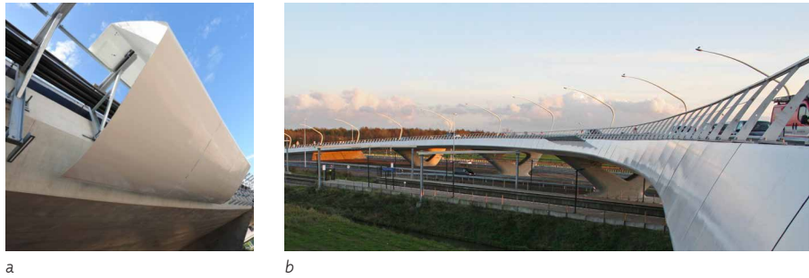
FIGURE 4.8 Installation and final assembly of the edge elements in the fly-over Waarderpolder. Royal HaskoningDHV, Joris Smits et al. (2012). Photo's by Ballast Nedam (2011).
