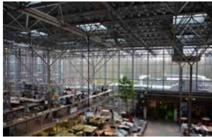
FIGURE 4.92 Realised steel space frame for the south-facing hall Faculty of Architecture TU Delft, 2017
