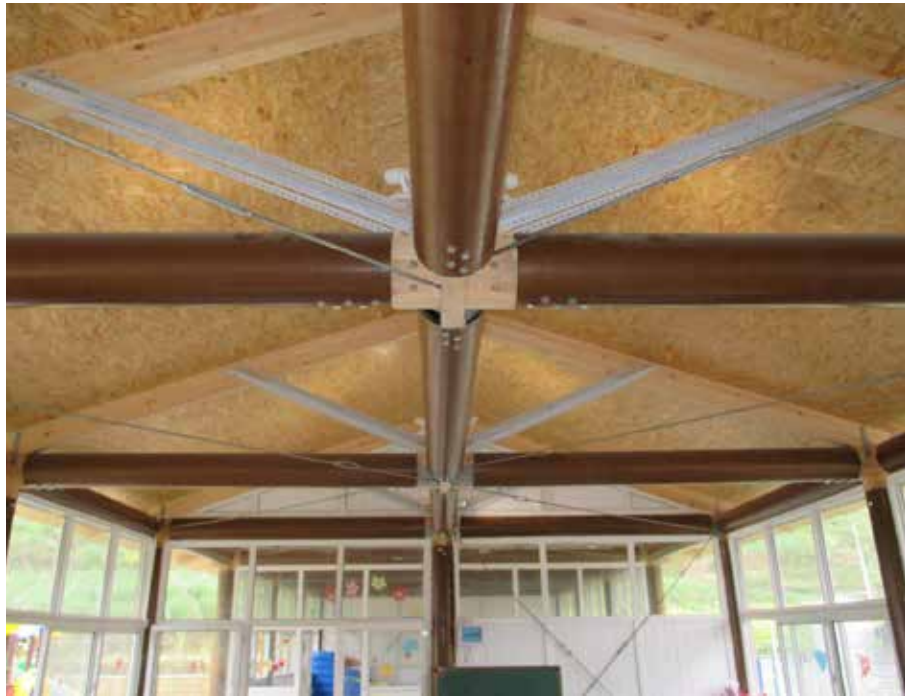
FIGURE 4.108 Paper tube, timber, perforated L-shape and steel bracing composition of the roof structure, 2014
