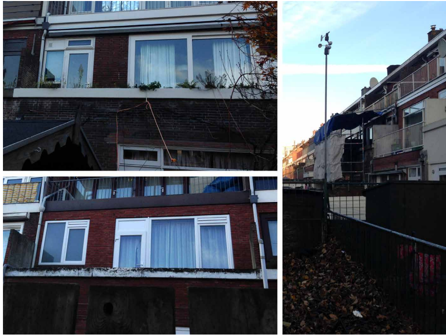
FIGURE 7.3 Maintenance problems in Oud Charlois, deterioration of balconies and façade. Source: author's pictures.
