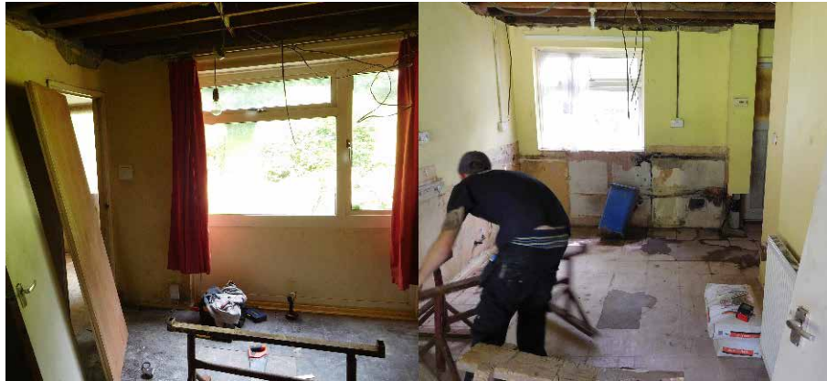
FIGURE 6.3 Ongoing void repairs. (Right: Notice kitchen removed in the far end.) Source: Author (June 2016).
