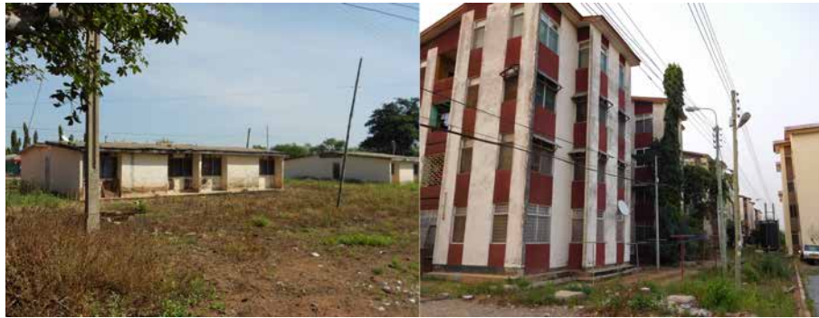
FIGURE 1.2 Rotten fascia boards, leaking roofs, and faded paint of some public houses.
