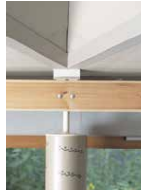
FIGURE 4.67 Westborough Primary School, detail of connection between the wall and the roof panels, 2001
