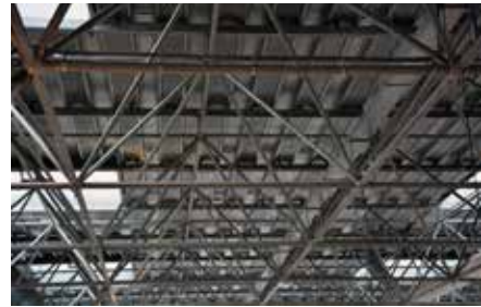
FIGURE 4.93 Space frame structure of the south-facing hall, Faculty of Architecture TU Delft, 2017
