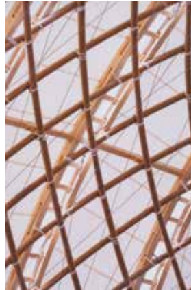
FIGURE 4.59 Detail of the connections between the paper tube lattice and timber ladder, 2000
