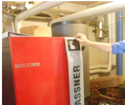
FIGURE 8.10 IEWAN: Collective pellet heater
